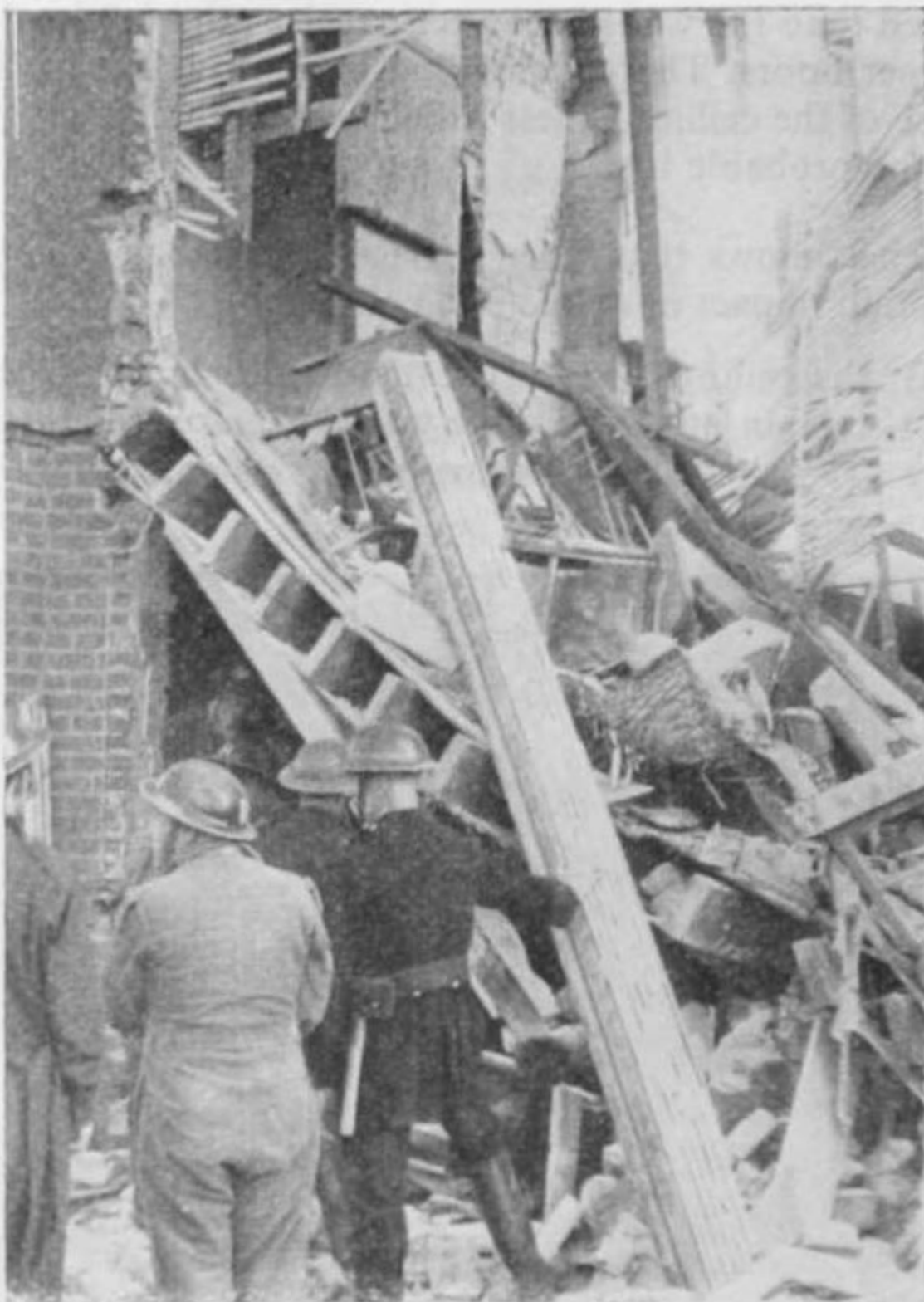
Fig. 79. Example of lean-to collapse (not in basement)
