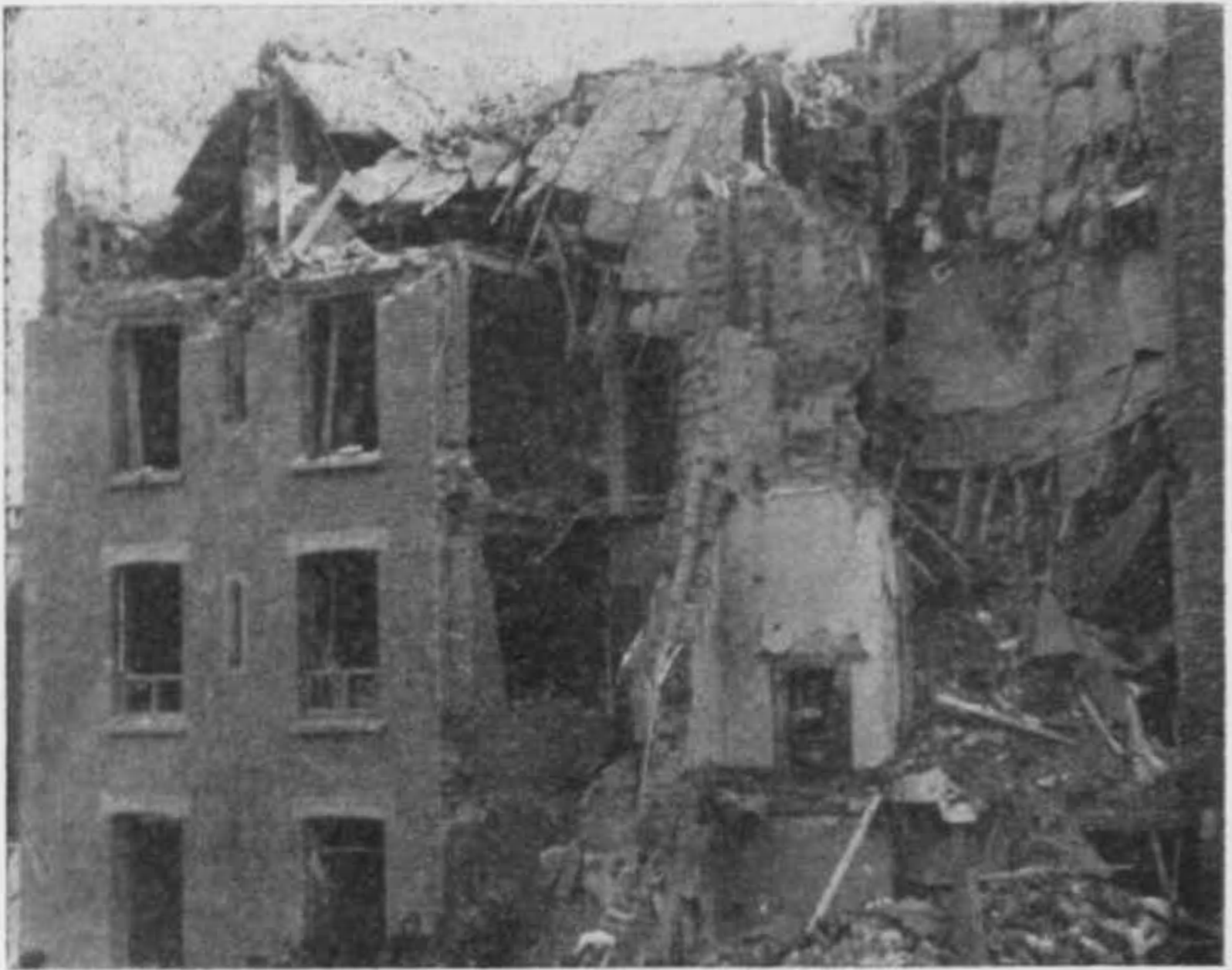
Fig. 7. Unframed building showing how walls support the floors (note collapsed concrete roof)
