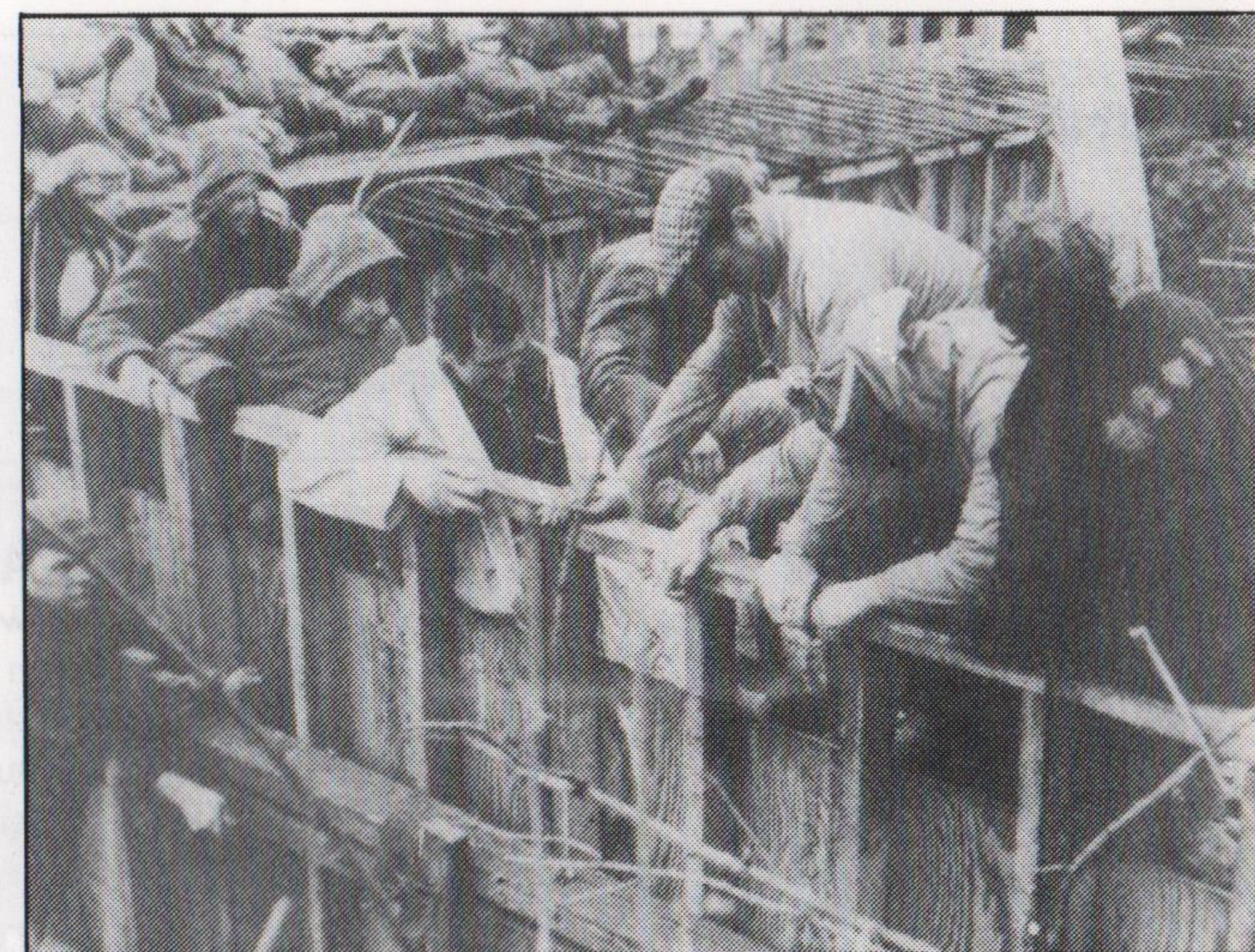
Peace campaigners obstruct contractors pouring concrete during the building of Mid-Glamorgan County Wartime HQ.
